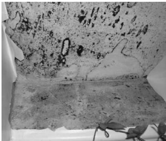
Fig. 1.6 Part of a bathroom ceiling where the paint has flaked away, revealing extensive growth and sporulation of sooty moulds.
